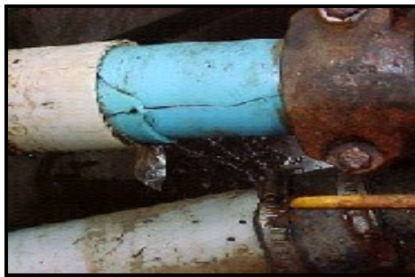
Flexible piping is cracked
