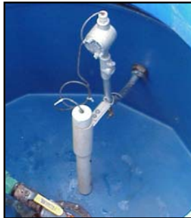
Float sump sensor
