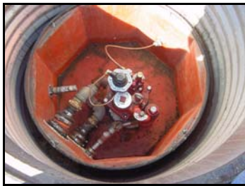
Dry, debris-free contained turbine sump
